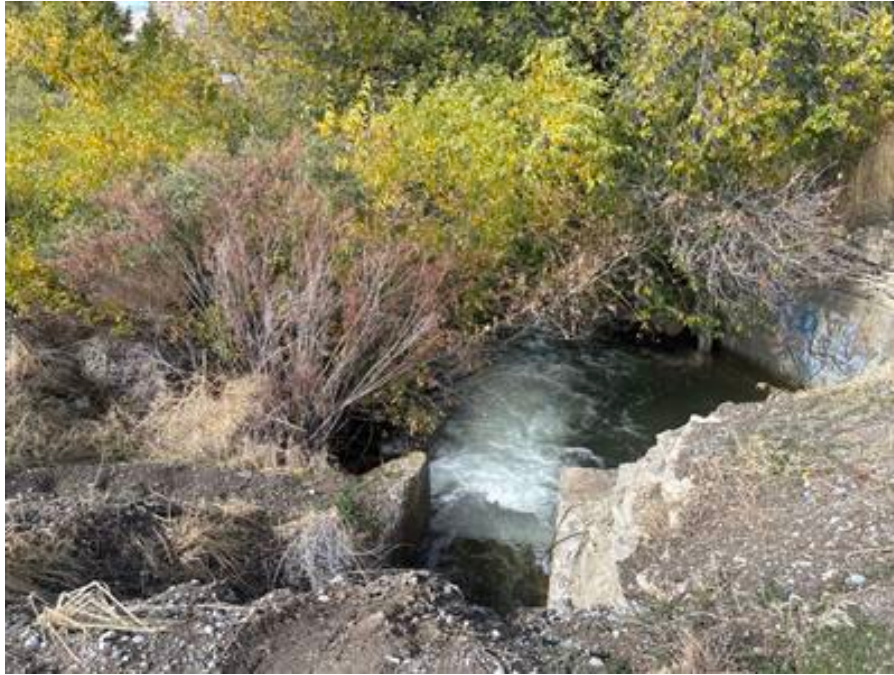
Photo of intermittent stream segment I-2b (location shown in Attachment B, page 17).
