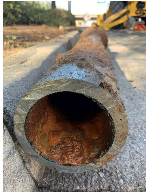
Example Pipe Tuberculation
